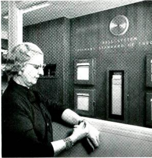
Principal frequency standard for the Bell System is this elaborately instrumented equipment at the Murray Hill, N. J., location of Bell Laboratories. Accuracy of this standard depends on the very precise vibrations of piezoelectric crystals.
