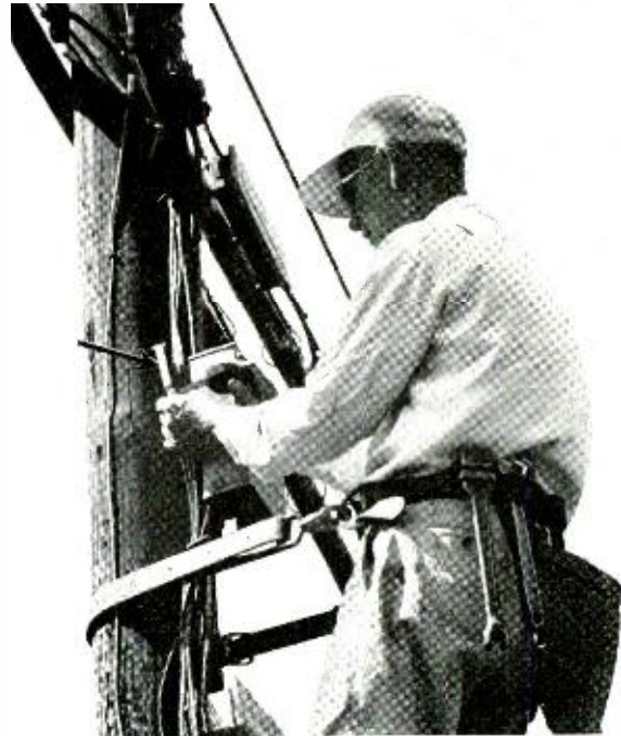
T. W. Rolph places B Drop Wire Cap (arrow) on disconnected wire.
