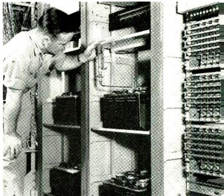
Fig. 4— J. E. Walsh, New York Telephone Company installer, makes a routine check of the batteries in an answering bureau. Over a dozen identifiers use a common power supply.
