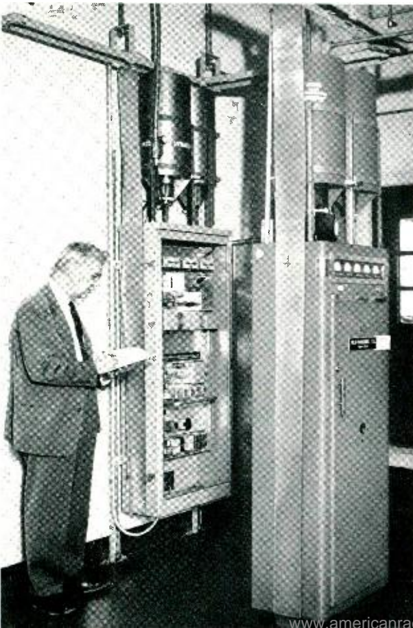
Fig. 2 — Engineer C. L. Garrett checks operation of the transmitter used in the trial. Transmitters for other mobile services are in the foreground.
