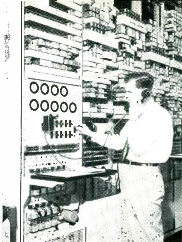
Fig. 3—The central office equipment provides break-in and control keys for technical operator A. L. Evans of the Chesapeake and Potomac Telephone Company of Baltimore City.
