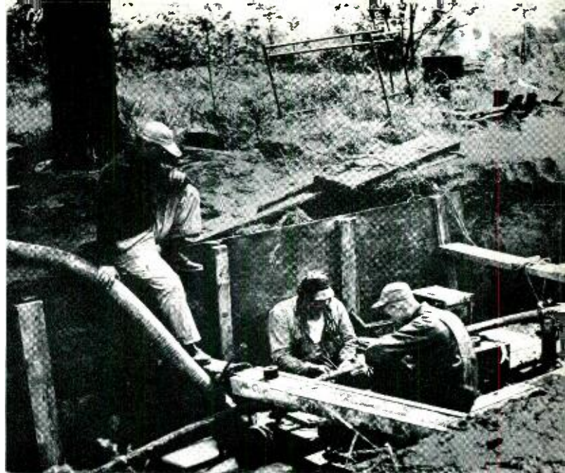
Fig. 6—Repairing a coaxial cable crushed by lightning that initially struck the tree at the left. Pumping was required to keep the pit dry during this operation.
