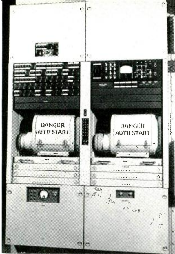
Fig. 1—Two bays are all that is required for the new ringing power plant.
