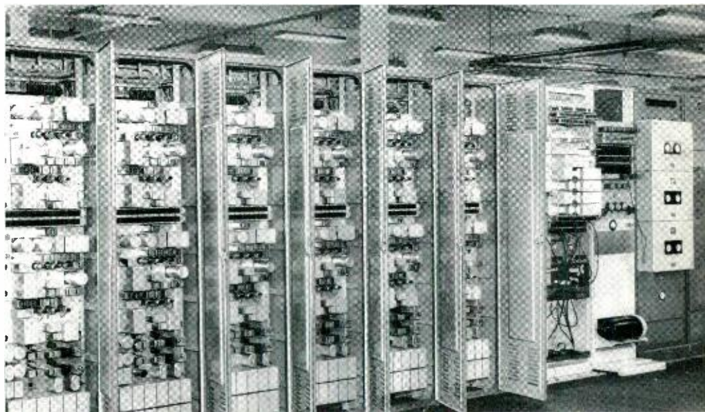
Fig. 4—The left-hand three bays contain conversion equipment for six additional channels. The other bays are conversion and temporary power bays used at Laurence, Mass., to simulate an existing six-channel system.
