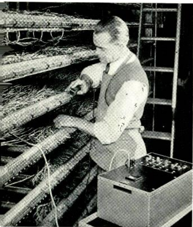
Fig. 1—The rapid line insulation test set in use in a central office.
