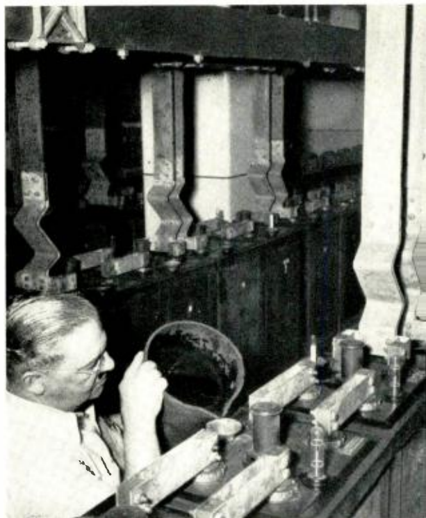
Servicing storage batteries in one of the larger type power plants used to supply several central offices in the New York area.
