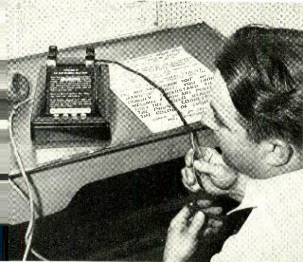
n New York City's Police Headquarters, an installer puts in a new key telephone. The four illuminated buttons of this red set indicate degrees of alert.
