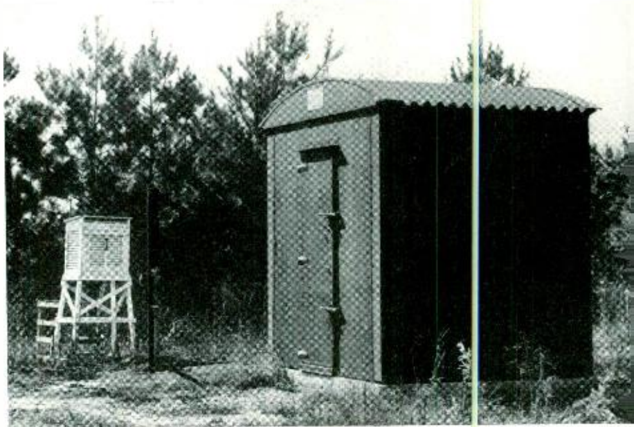
Prefabricated metal hut for coaxial auxiliary repeater equipment with double cellular wall panels. The outer walls are filled with insulating material and the inner ones with dry sand
