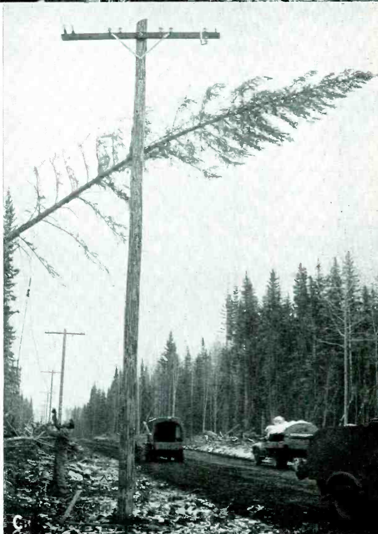
C—The soil formation along much of the Alcan Highway consists of a few feet of muskeg—a composite consisting chiefly of decayed vegetable matter—resting on perpetual ice. As a result, the trees are shallow rooted and fall with very little urging. As many as 33 trees have been removed from the line in a single day over one section. The high-strength steel wire employed prevents such falls from breaking the wires, but short circuits are caused and are promptly removed by patrolling line crews
