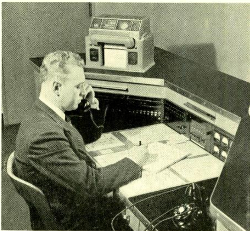
To insure continuity of the numerous services at Murray Hill, such as electricity, water, compressed air, and ventilation, an automatic alarm system is installed that gives immediate indication of any condition that should be remedied. These alarms, as well as the fire alarms and the watchman reporting system, are all brought to this desk at the Control Center
