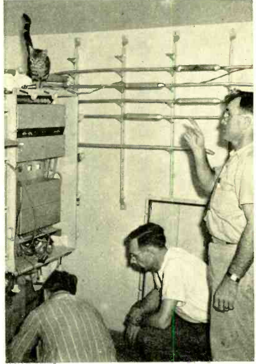
In the Key West cable hut, C. A. W. Grierson (center) watches the submarine cable being strapped in place. Also pictured are representatives of the A T & T and Southern Bell, and the local mascot
