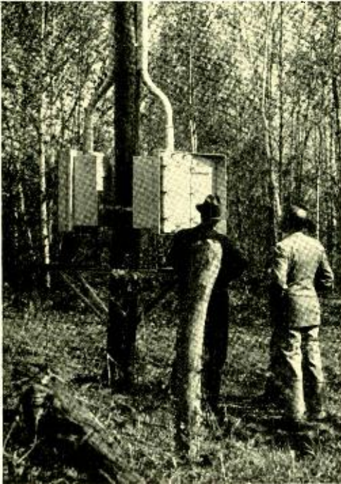
Fig. 4—At some locations the repeaters are mounted directly on the poles
