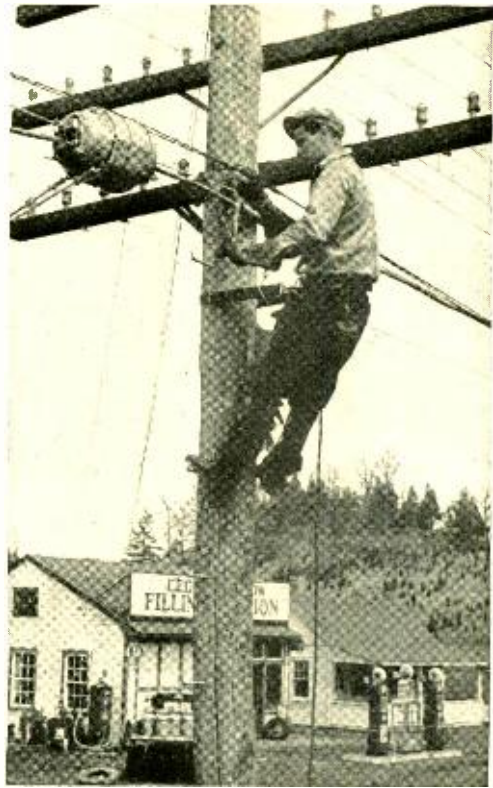
Fig. 2—A telephone lineman dead-ending the lashing wire at the pole. The lashing machine is shown at the left and is in position to begin lashing the next span of the cable
