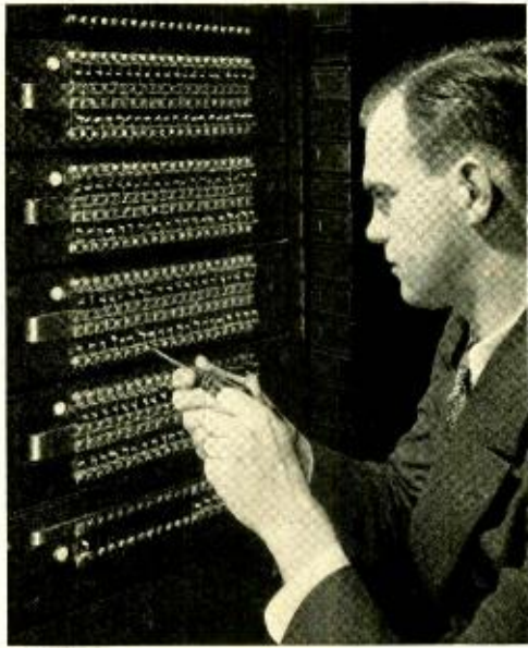
Fig. 1—J. Michal is shown replacing a blown alarm fuse. These fuses flip up a small glass bead as a visual signal and ring a gong at the time they blow
