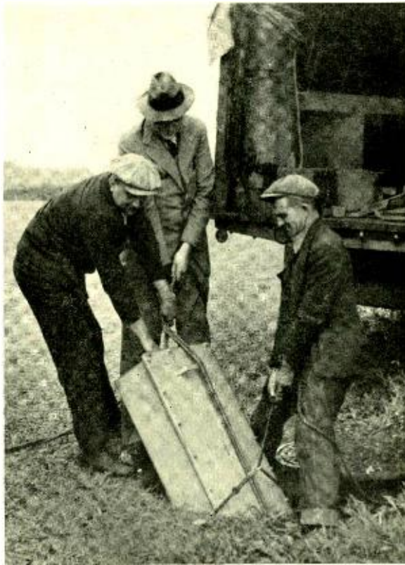
Fig. 6—Lowering a repeater into manhole E, some ten miles south of Trenton
