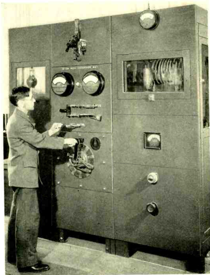
Fig. 5—The fifteen-kilowatt oscillator employs a manually operated tap switch for adjusting the output
