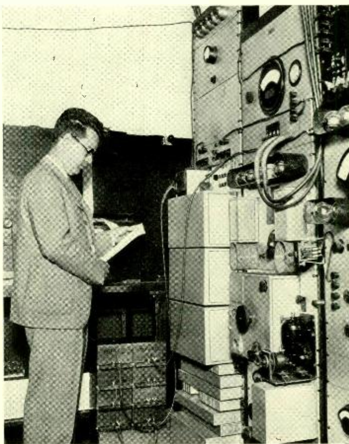
Fig. 1—The new recording transmission measuring set consists of two bays of equipment, one supplying the testing voltage, and the other measuring the insertion loss of the equipment under test
