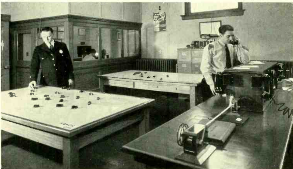
Fig. 1—Radio dispatching room for the Newark police system. Left to right: Lieutenant William Sacher; Samuel Cobb, Dispatcher, in booth, and Robert Schweitzer at the switchboard
