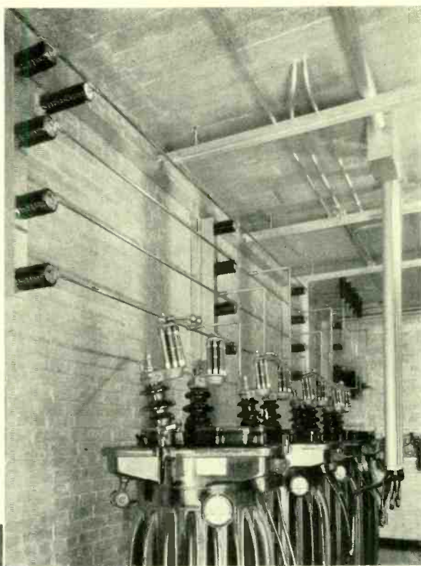
Fig. 4—13,000-volt transformers and busses supplying the high-voltage rectifier. The upper bus is the 17,000-volt direct-current supply
