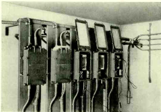
Fig. 6 — Terminal boxes in the Key West cable hut
