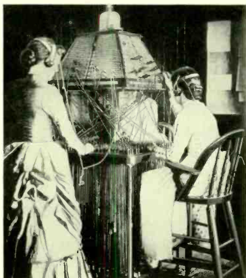
Fig. 3—Plugs and connecting cords as they appear in the Law board of 1882
