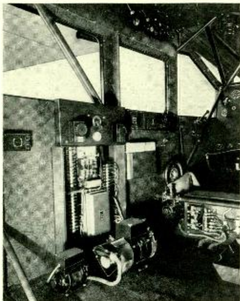
Interior of Fairchild plane showing radio-telephone control equipment
