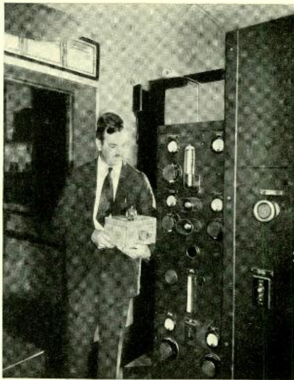
Fig. 2—A corner of the operating room at station WOC, showing a part of the radio transmitter at the extreme right with the D-90684 Oscillator-Amplifier mounted adjacent to it. G. D. Gillett is holding the crystal oscillator and constant temperature oven, and over his head to the left is the loudspeaker on which the program for the monitoring station is received
