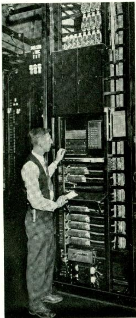
Fig. 1—An attendant is here shown operating one of the control keys of an automatic incoming-selector test frame
