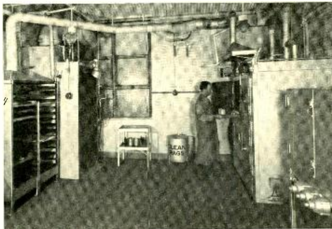
Fig. 3—The japan room. Left to right: drying rack, small spray booth, baking oven (into which Charles Stone is placing equipment he has just sprayed), and crystalizing oven. Exhaust systems are coupled to all these units
