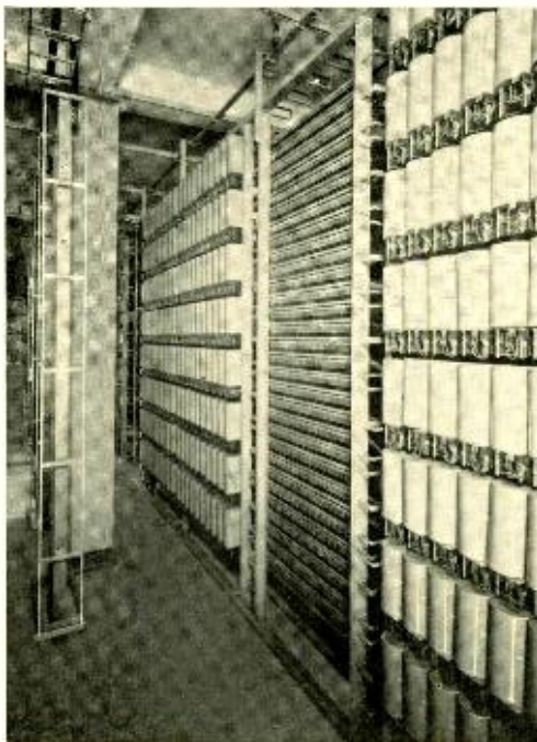
Fig. 2—Selectors are mounted twenty on a shelf, and two groups of eight shelves are arranged on one frame with cross connecting terminals between the groups
