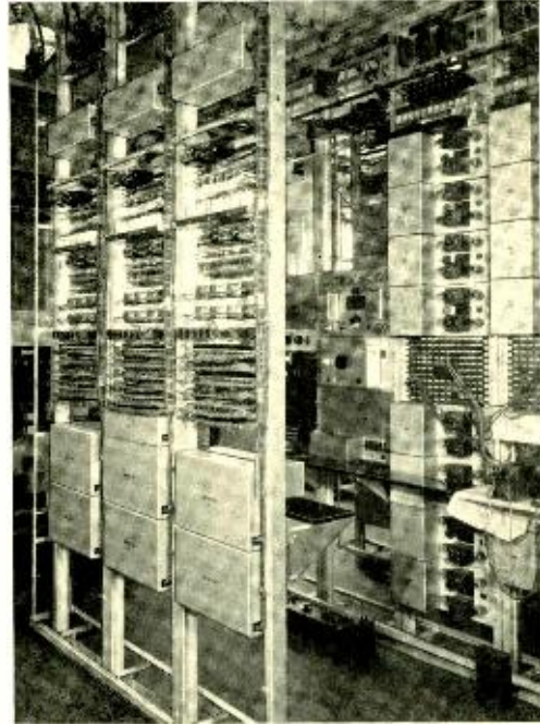
Fig. 3—General view of vodas relay and telephone repeater equipment at Walker Street, taken during installation and test
