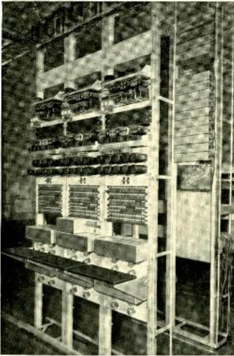
Fig. 1—Vodas relay equipment at Walker Street
