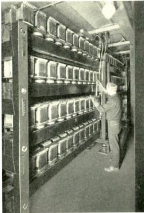
One-twelfth of the battery. These two racks, like all the others, hold eighty-eight cells each
