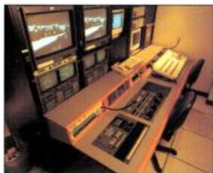
Camera control supports four DVM-500 studio cameras.
