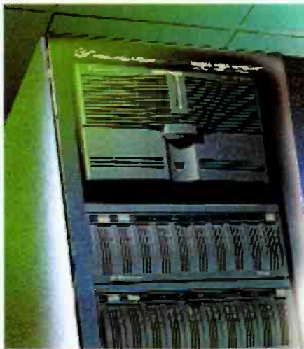
GVG server products will play a role in NBC's new centralcasting facility based in New York.
