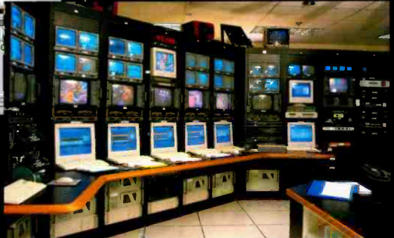
Ackerly's Central Casting system in Salinas, CA uses Sundance technology
