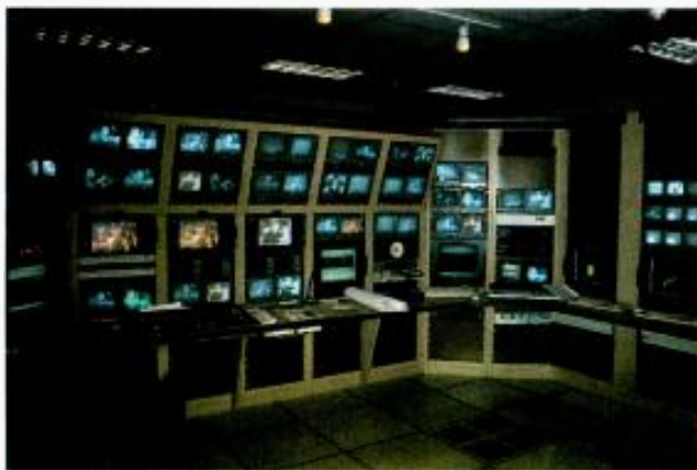
The control room at WWOR-TV Secaucus, N.J., handles all satellite recordings with the help of Floral automation.
