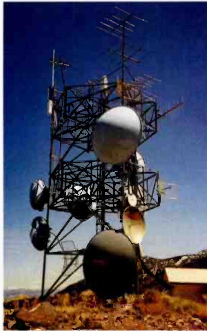
One of two translators used in the test, this one is located in Cove, Utah, 67 miles from the first site.
