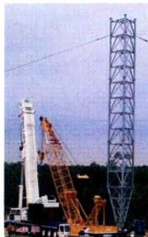
A SpectraSite crew sets the base for the 1.9 million-pound Mobile, Ala., tower.
