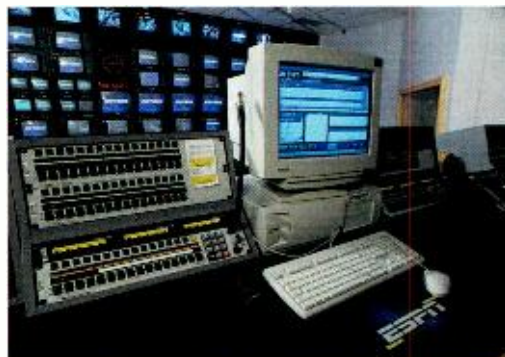
Production Control Room #9 is the nerve center for ESPNEWS.
