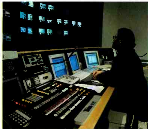
WNET now occupies two floors instead of 10. Master control is shown above.
