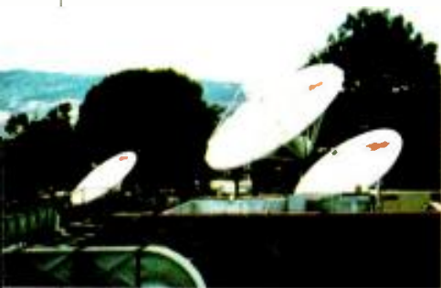
RCN-TV's uplink site in Bogota, Colombia, is outfitted with Andrew Corp. 7.3-, 4.5-, and 3.6-meter C-band earth station antennas.
