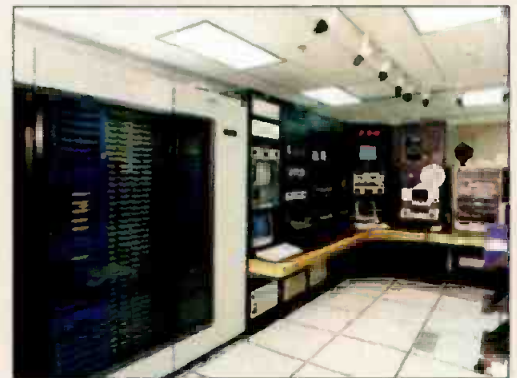
Communications Engineering Inc. completed this new digital origination facility for BET Jazz.
