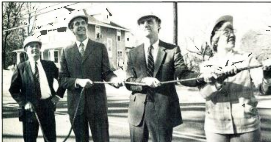
String that cable. Tribune-United Cable of Montgomery County (Md.) has begun construction of a three-hub system that will ultimately reach 220,000 homes in the sprawling Washington suburb. On hand to launch the build by pulling cable through the first utility pole: John Schmuhl, vice president and general manager, Tribune-United; David Scull, president, county council; Charles W. Gilchrist, county executive, and Viola Hovsepian, Rockville (Md.) city council member.
