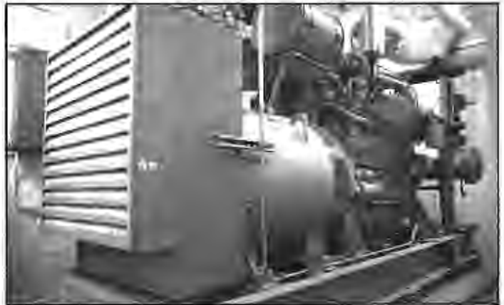
At the bottom of it all: a 450 kw emergency generator capable of keeping the ABC Washington news operation on the air for one week.
