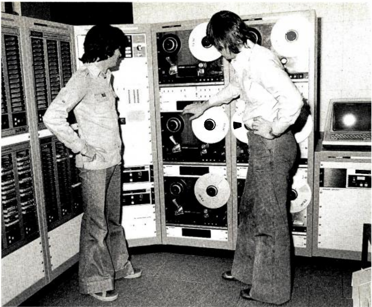
Graeme Greenwood, Audio Broadcast Services Engineer and Warren Gillispe, Program Director of 6KY inspect the new 903E.
