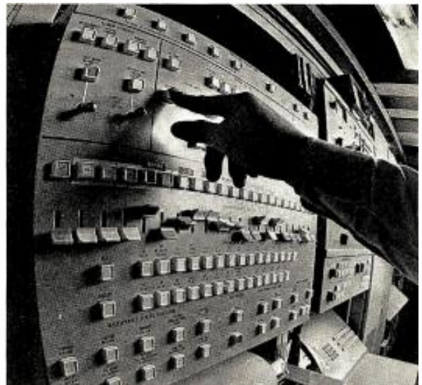
Electronic switching systems, now in wide use, provide high speed and flexibility for the nation's telecommunications needs.
