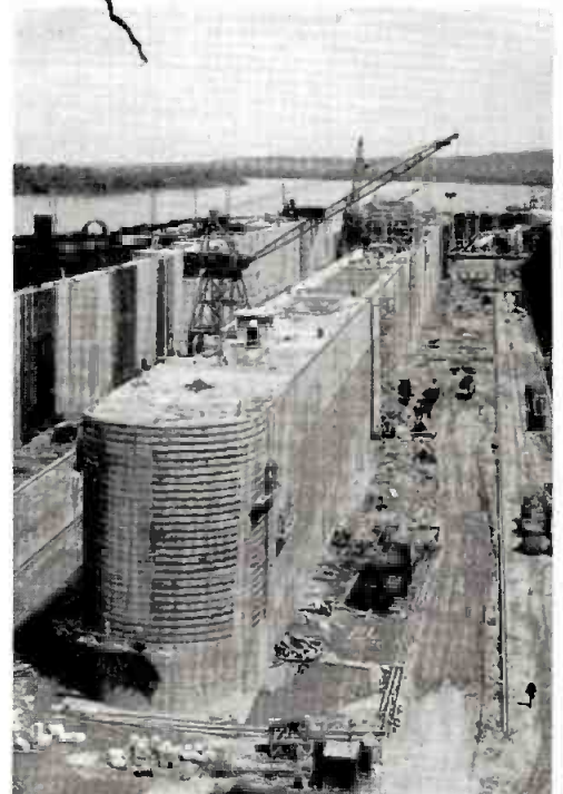
Construction view of Markland Lock and Dam — one of several under construction to handle tows longer than Queen Mary — as wide as a carrier.
