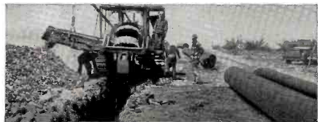
Goodbye Gas Shortage. For years now, gas companies have been rapidly laying new pipelines to ease the gas shortage. The job has been made easier with this giant trenching machine made from USS MAN-TEN Steel. MAN-TEN has such high strength that the machine can be made stronger and lighter than with carbon steel.
