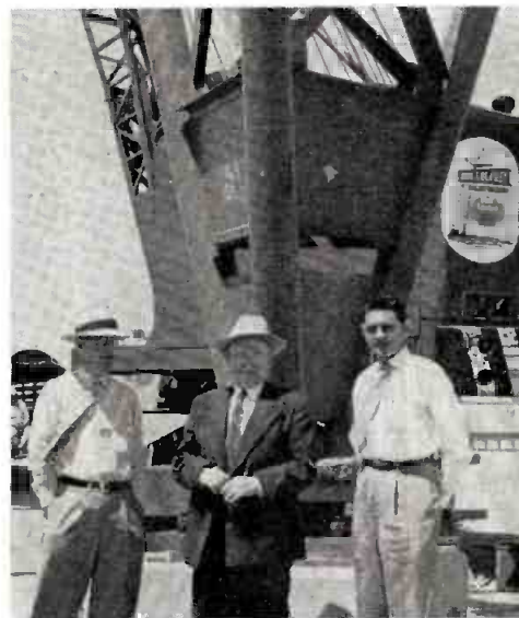
BASE SECTION of what is to be Texas' tallest tv tower—1,113-ft. above ground—is inspected by WBAP-TV Fort Worth officials (l to r) R. C. Stinson, director of engineering; Harold Hough, vice president of Carter Publications and director of WBAP radio and tv, and Bob Gauld, program director. Completion is scheduled Aug. 1.
