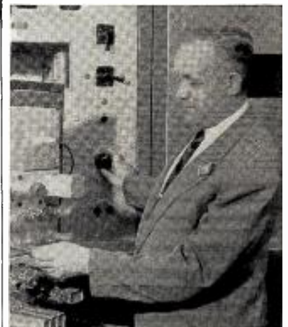
Bob Millham inspects the external equipment required to convert a General Electric 35 KW VHF transmitter.
