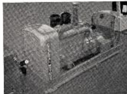
WKTV—UTICA, N. Y., uses a 100 kw. General Motors Diesel generator set for stand-by power. Set can be started remotely from the control room. Low vibration characteristic of engine permitted installation in room adjacent to transmitter and within 30 feet of studio.
