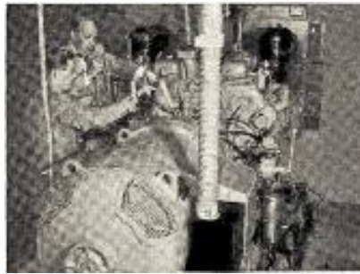
WJR—Detroit, Michigan, uses 200 kw. GM Diesel generator set as stand-by power for 50,000-watt transmitter. Compactness of unit permitted installation in garage adjoining transmitter building—eliminating cost of a specially designed building.
