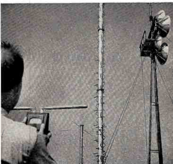
G-E HELICAL ANTENNA TEST. A field intensity test is run on a four-bay helical antenna installed at Electronics Park. The helical antenna, used with all UHF transmitters, boosts Effective Radiated Power up to 20-25 times.
