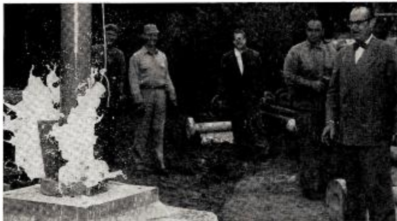
GALLON of Wisconsin milk splatters against the first column of a new 1,032-ft. tower being erected by WTMJ-TV Milwaukee. Christening new tower is Walter J. Damm (r), vice president and general manager of radio, Journal Co., station licensee. Workmen were not identified.
