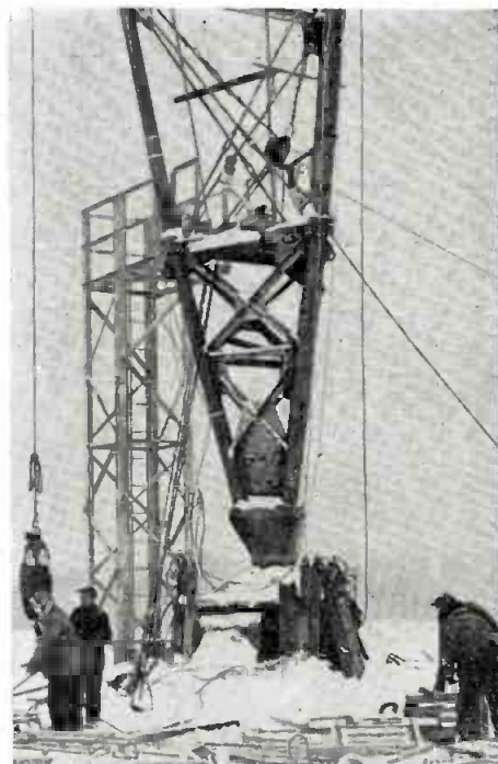
A construction photograph shows giant tower's base. More than 1400 cu. yds. of concrete was used to form base pier and guy anchors.
