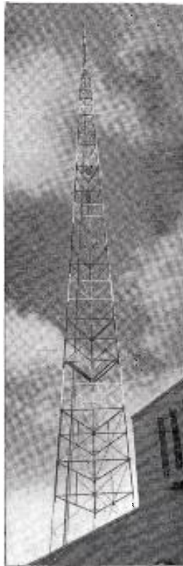
WOW, Omaha, Nebr., Truscon Self-Supporting Radio Tower, 500 feet high overall.
