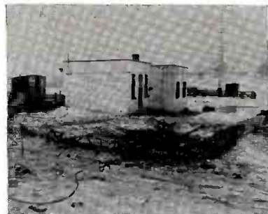
PART of one of the 320-ft. towers of WPPA-AM-FM Pottsville, Pa., which collapsed during a recent ice and wind storm, lies near the AM transmitter building. The building was missed by the falling structure. Using another tower, WPPA was back on the air within 45 minutes, station officials reported.
