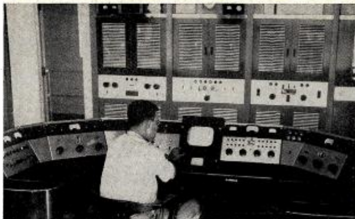
THIS COMBINATION console arrangement has been installed by WKY-TV Oklahoma City, which will begin commercial operations by mid-May or early June, according to P. A. Sugg, station manager. Console enables an engineer to control the television, FM, AM and auxiliary broadcast signals. Horace Merriman, transmitter supervisor, is testing the television monitor and controls in the center of the board. At left are the auxiliary transmitter controls. FM operations are at the right of the panel. Ninety percent of the TV transmitter installation is now complete.
