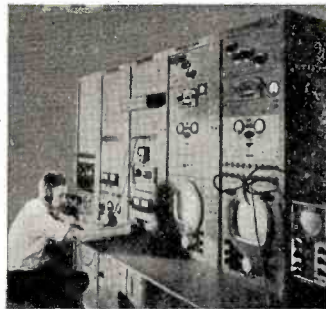
G-E transmitter monitor control board.
