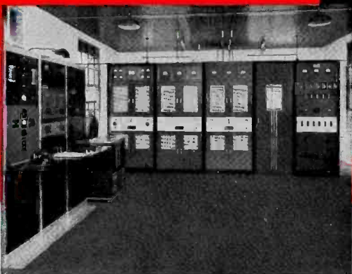
Shown here is RCA 5-D installation at Station WBRC.
